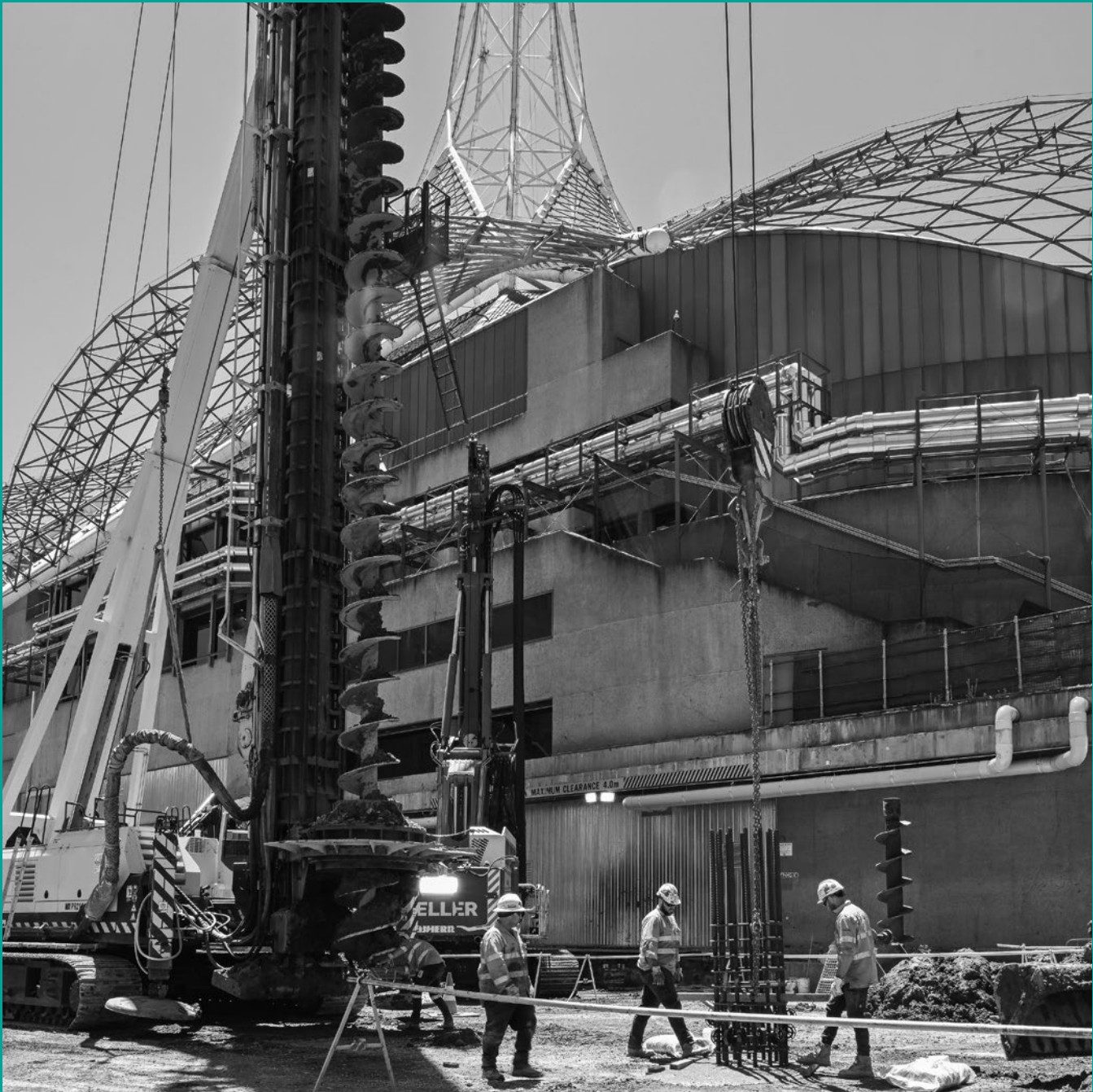
Piling underway at the back of the Theatres Building. Photo courtesy of Keller.
