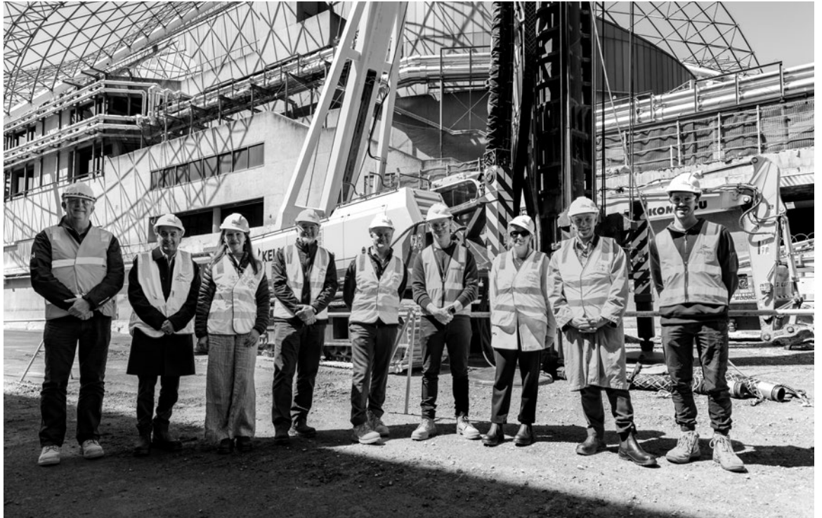
Members of the Victorian Arts Centre Trust tour the construction site with representatives from Development Victoria and Lendlease. Photo: Mark Gambino.
