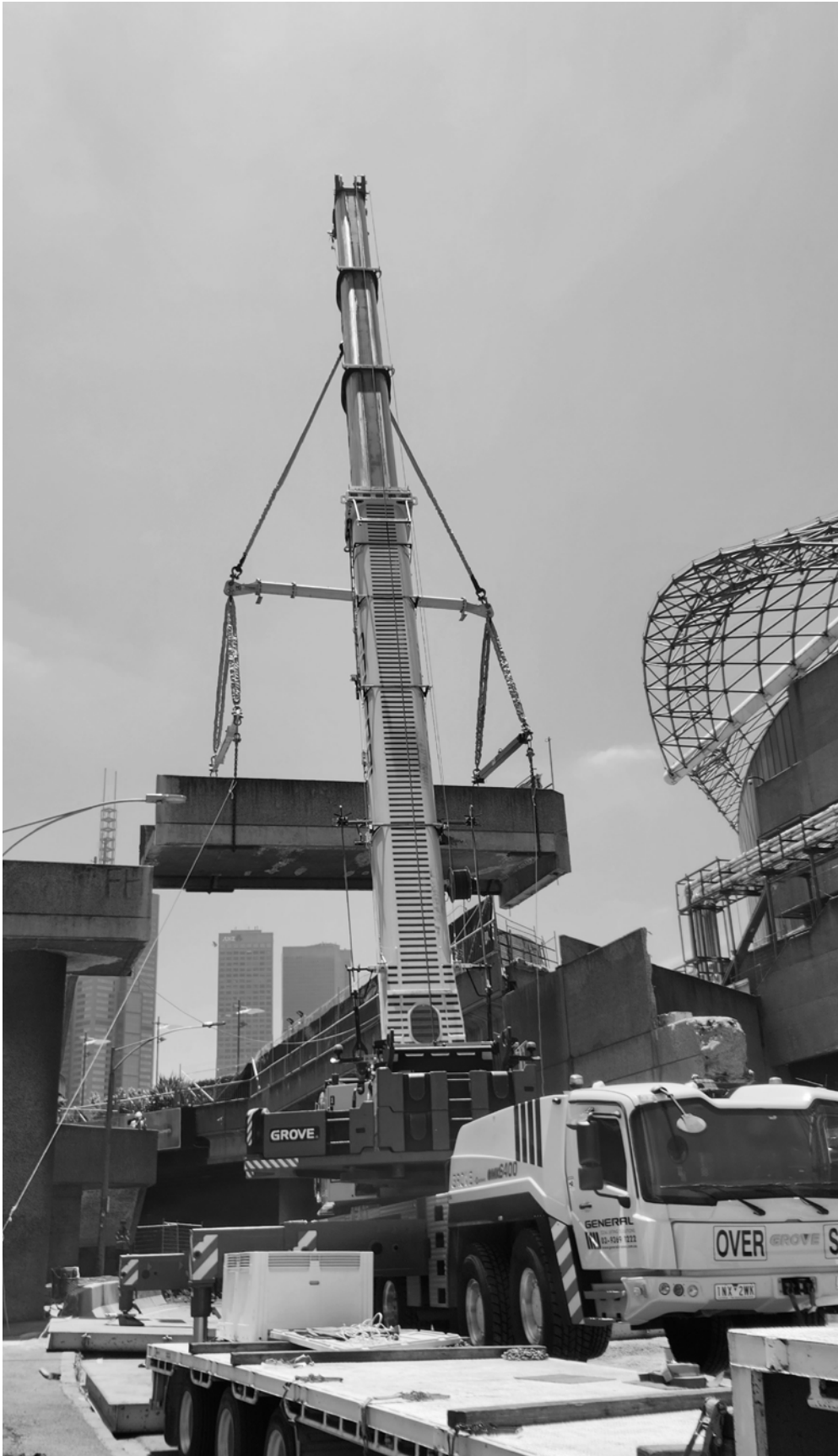
A concrete bridge spanning Sturt Street between the Theatres Building and City Road is removed in January 2023.
