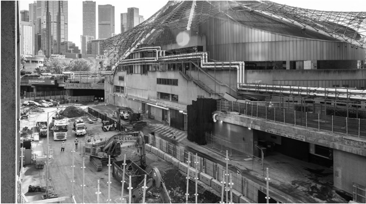
Construction at Arts Centre Melbourne, with above-ground pipework seen on the Theatres Building façade, and construction works continuing at Sturt Street level.
